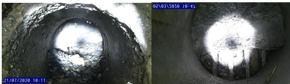
Examples of blocked pipes
